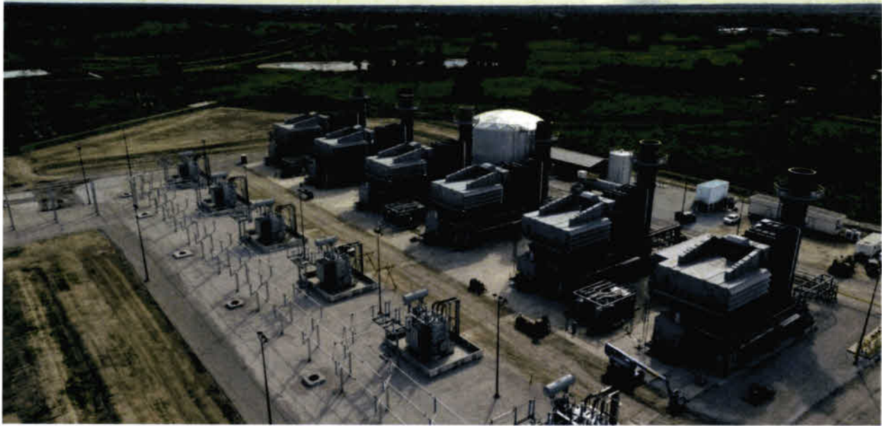
Figure G-3. Example LM6000 Pro Energy Units
