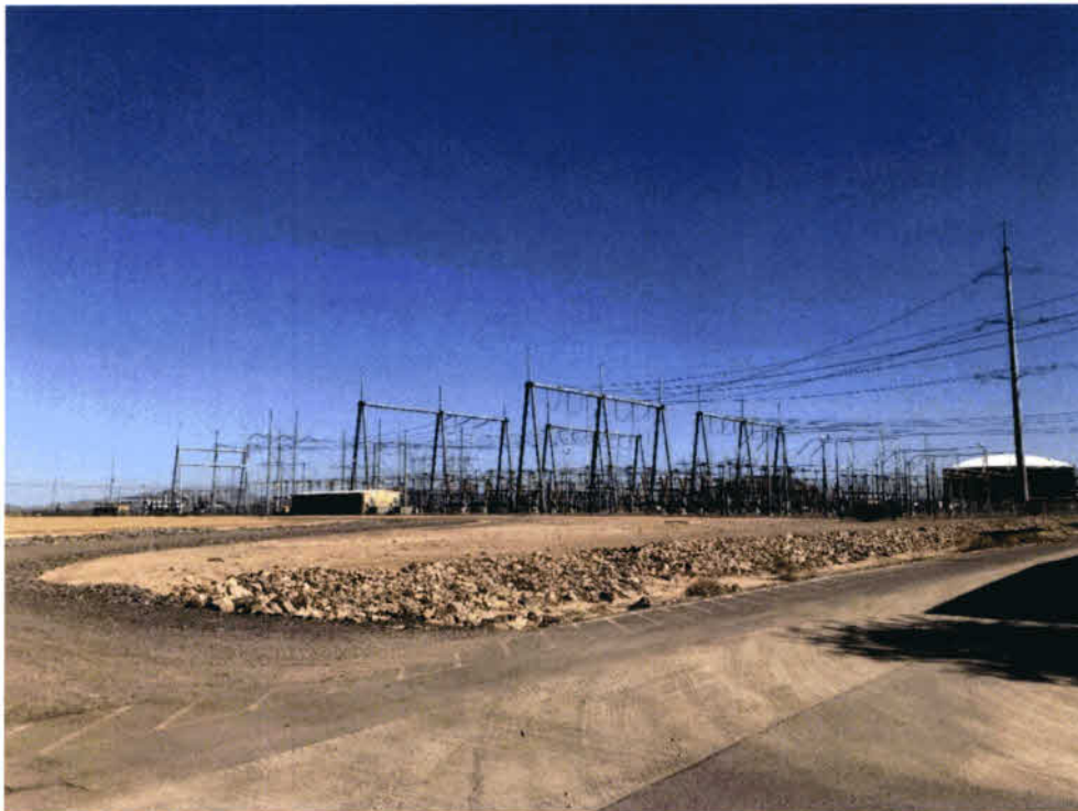
View of existing Redhawk Switchyard looking northwest.
